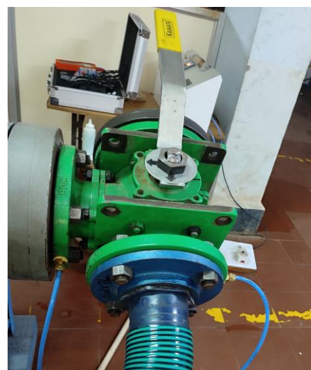
Fig 3.1.4 Differential Pressure gauge mounting on inlet and outlet of 3way ball valve
