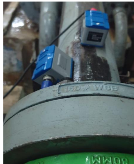
Fig3.1.2 Ultrasonic Flow Sensor Mounted on Pipe
